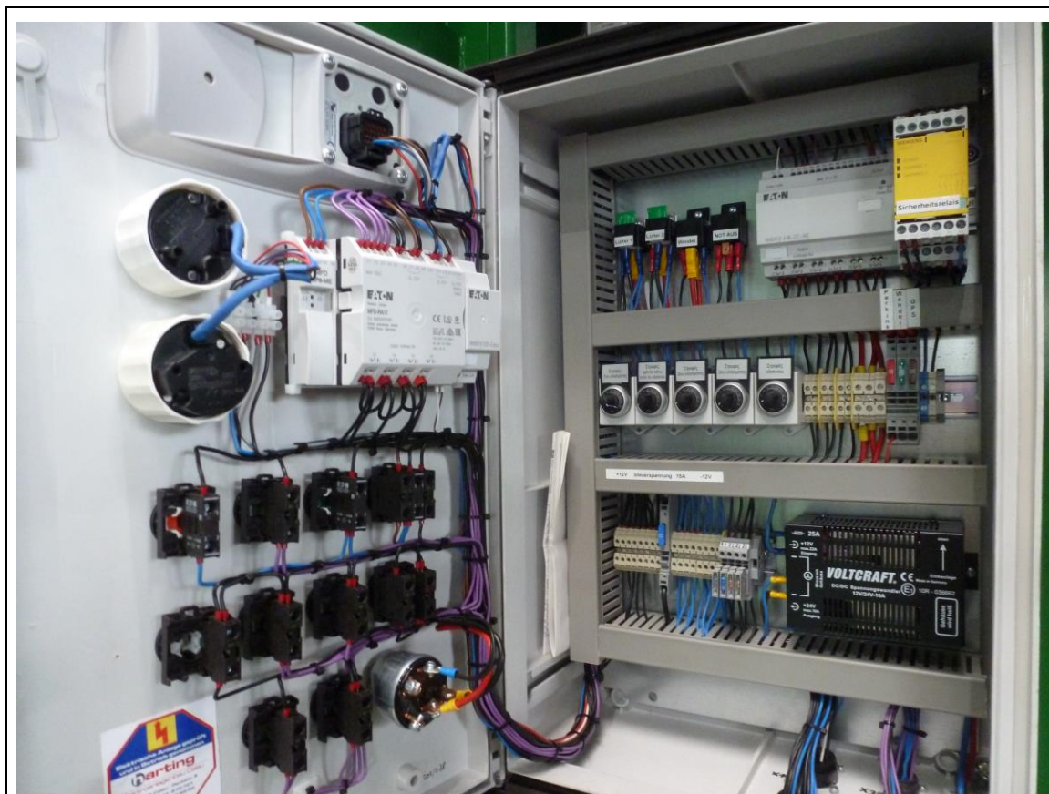
fig. 8-8: Control unit in the control cabinet
