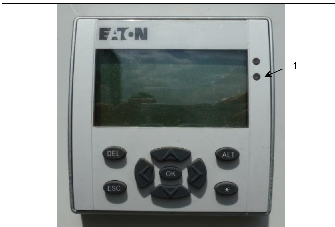
fig. 4 – 6: Monitoring of the hydraulic system
